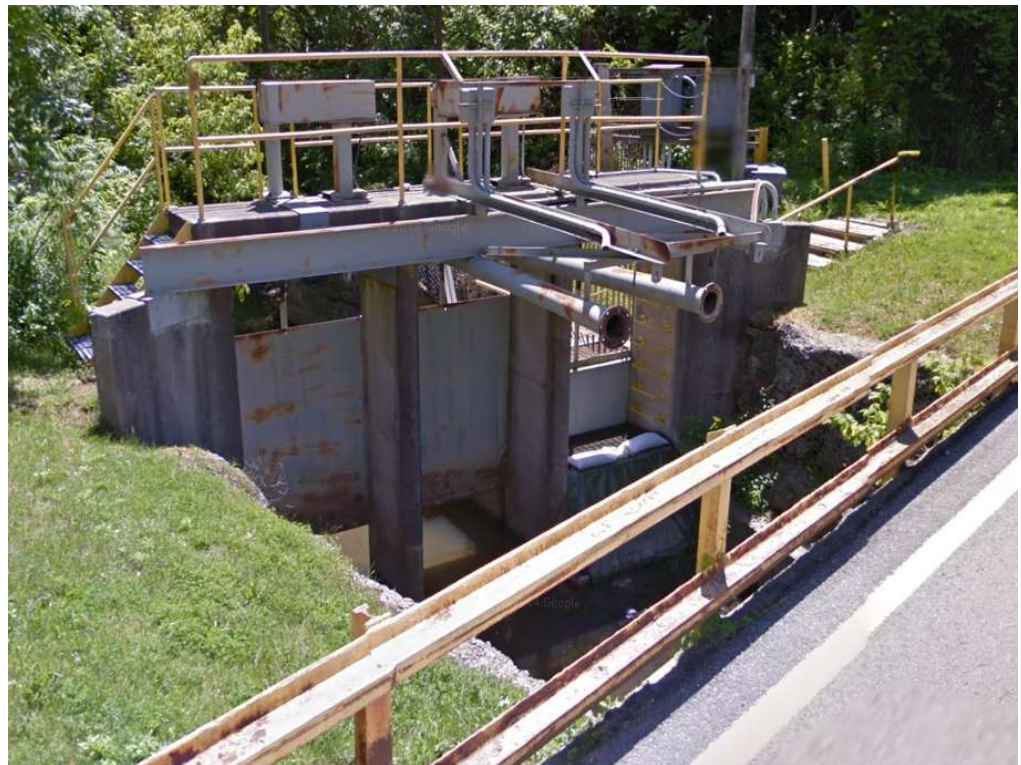
Figure 23 Wignell Control Structure - 01
