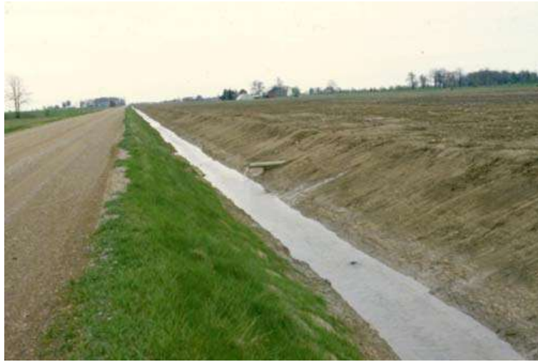
Figure 5 Example of clear drain
