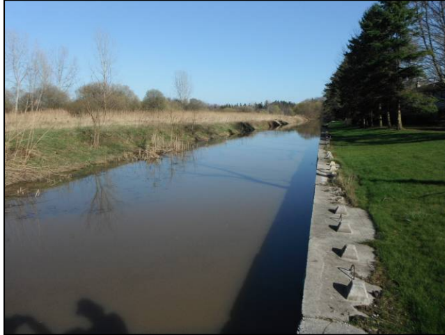
Photo 11: Reach 8-WM, channel character and hardened edge (emergency erosion protection works constructed circa 2008)
