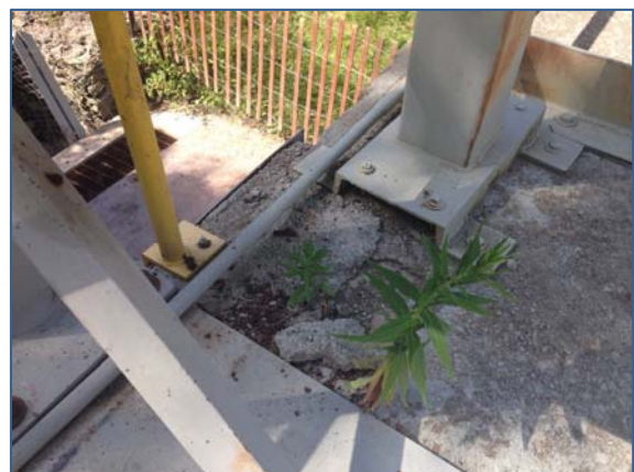
Figure 3: Localized Concrete Spall
