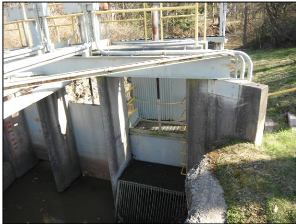
Photo 12: Reach 9-WM, water control structure at Lakeside Road
