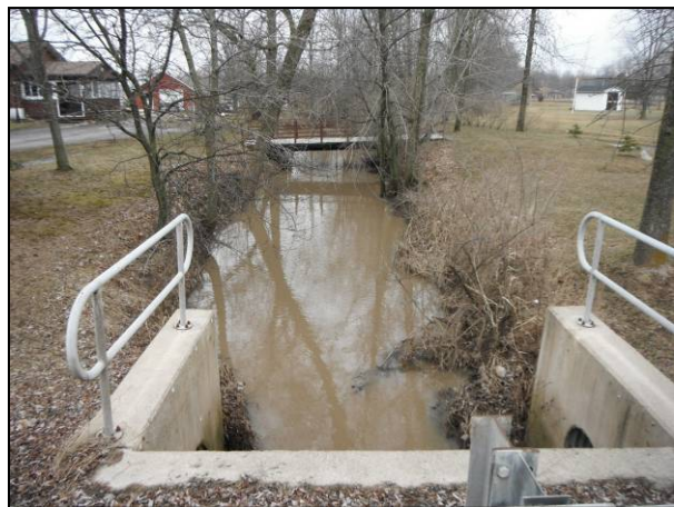
Photo 48: Reach 6a-B, Hwy # 3 culvert crossing headwall & lateral drainage (piped roadside ditching)pipinginterface. Former Geo. A. Schooley Award Drain.
