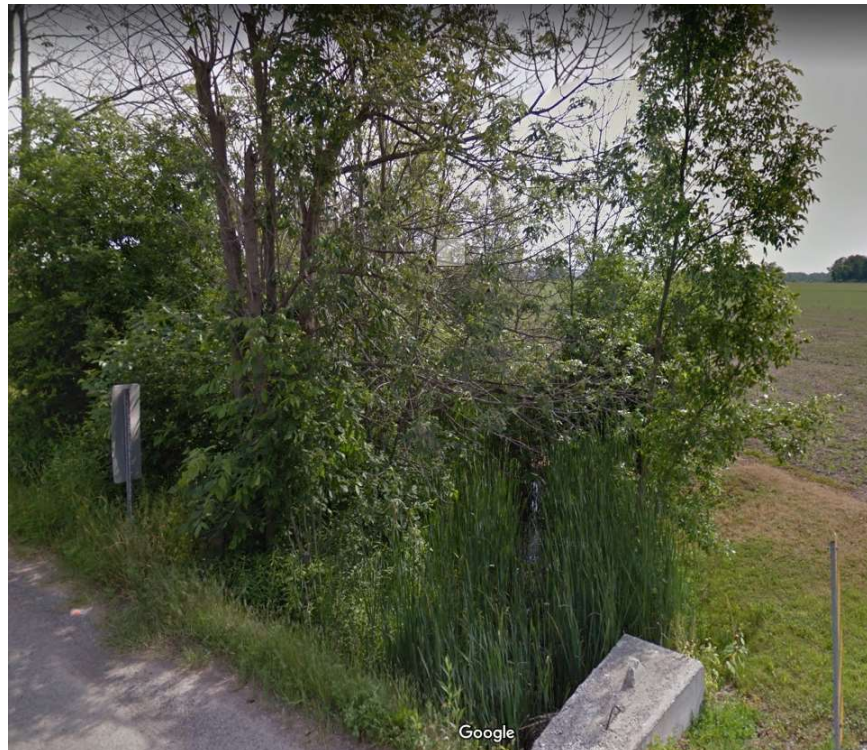
Figure 6 Obstructed drain; Wignell @ East side of Weaver Road This flow is obstructed by tree growth within the banks. Bull rushes provide evidence of standing water. The expected performance of the culvert based on this approach is compromised and unlikely to perform as designed or expected.
