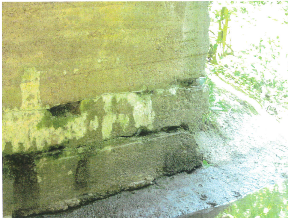
Large cracks on the north end of the west abutment wall
