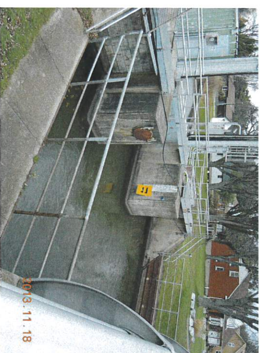
Eagle Marsh Drain flood gate.
